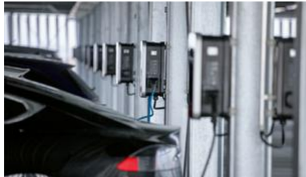
Electric charging station in Ditzingen parking facility
