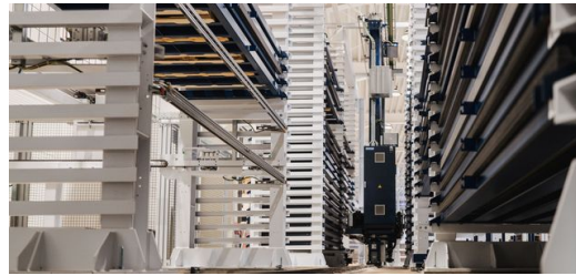
The large-scale storage system: STOPA sets the sheet metal on its production journey entirely automatically – and retrieves the finished parts with the same level of efficiency.
