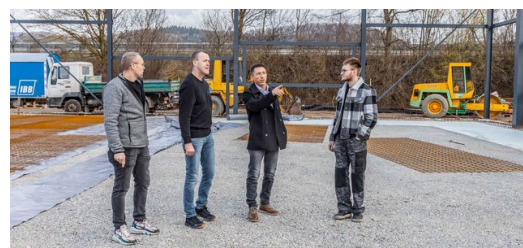
DELO is planning on relocating to neighboring Hechingen in September 2023. Construction work is in full swing. With a developed area of 2,000 square meters, he is aiming to more than double production compared to
