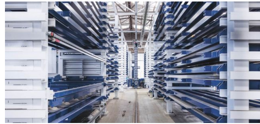
<p>Freighter Group has had no luck with previous attempts to automate processes. This is set to change with the new equipment. This includes an automated storage system.</p>
