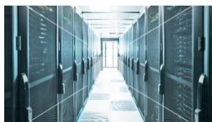
Picture 1: Data center
